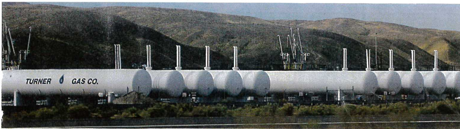
Turner Gas' propane rail terminal in Carlin, Nev.
